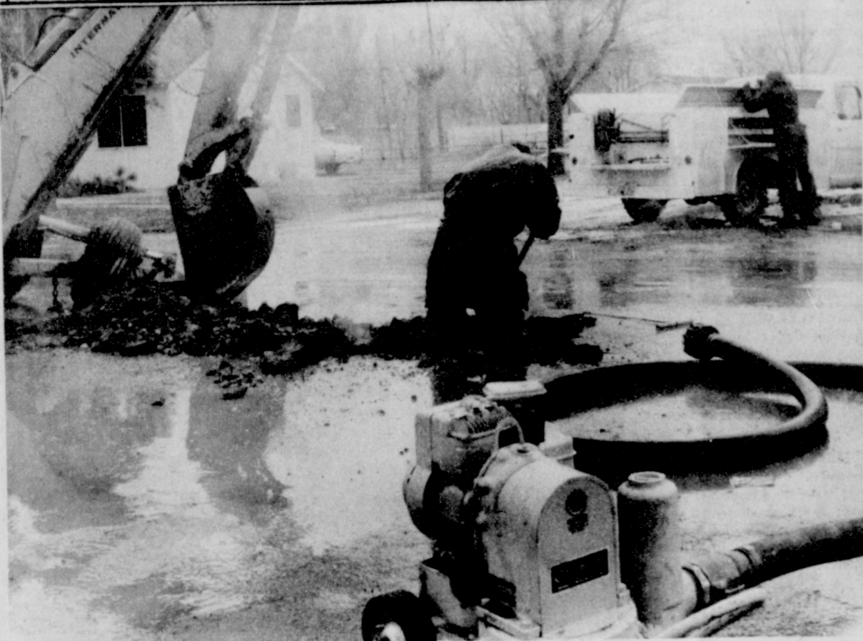
Scenes like this may become somewhat numerous in the next several weeks as Spearman City work crews repair broken water mains. The mains, in many cases have frozen as a result of the protracted cold spell. The thawing process sometimes results in a break.
