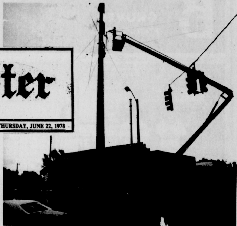
Community Public Service's $15,000 corner pole, is a monument to progress in the Spearman area. The new pole is anchored in 24 ft. of cement, and will handle the load of the main lines now attached to the pole.
