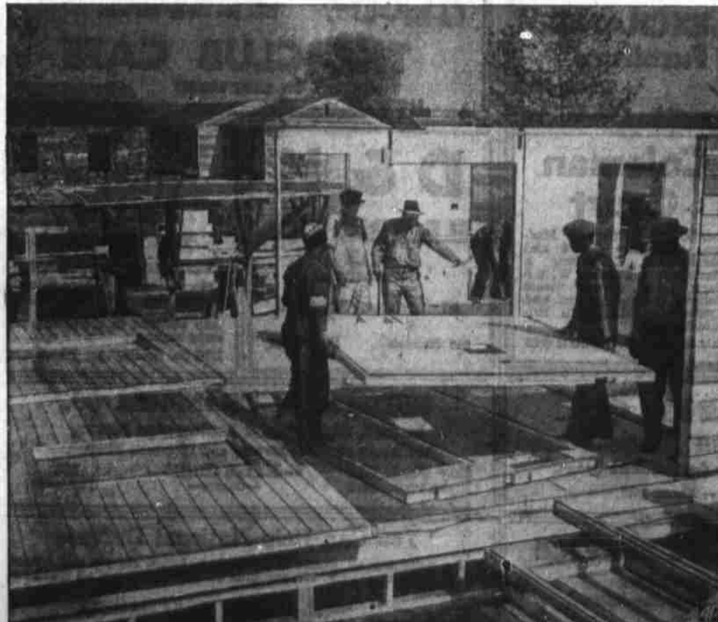
INSTALLING WALL PANELS —Workmen installing an interior wall panel in a structure of a war housing project at Hampton Roads, Va. Prefabrication is reported to be saving time.
