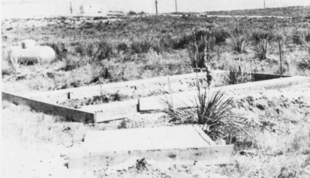
FOUNDATIONS POURED . . . The anchor points and foundations for the new law enforcement radio communications tower, located one half mile south of town off Highway 214, have been poured and now await actual construction of the 300 foot tower and a metal building. An auxiliary generator will be located on the site and will kick on in the event of a power failure to enable constant radio communication by law enforcement agencies. The project is a city-county endeavor with the South Plains Association of Governments being the coordinating agency for federal funding. The federal government will pay 75 percent of the total cost with the city of Muleshoe and Bailey County sharing the remaining 25 percent of expenditure.
