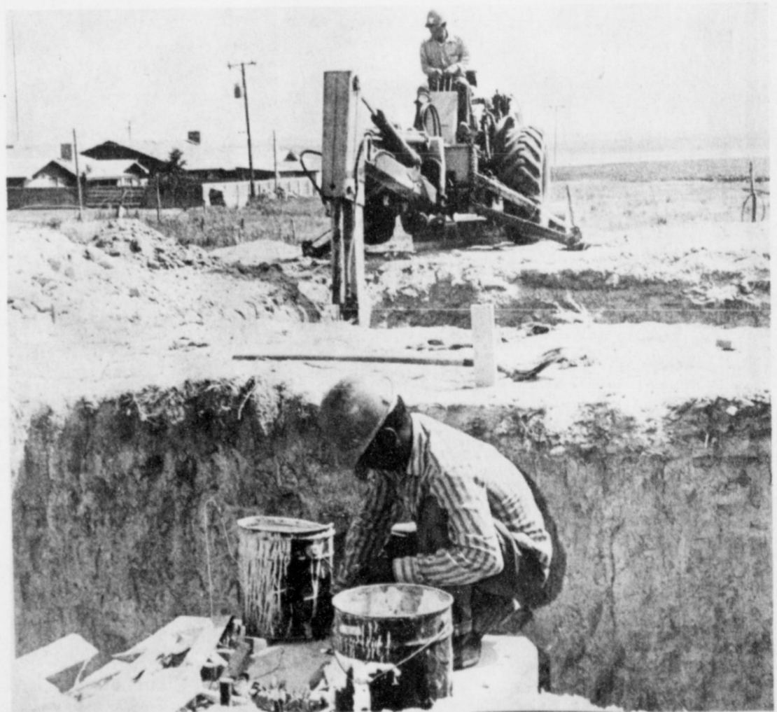
ELEVATED WATER TANK . . . Workmen were "hard at it" this week, beginning construction of the foundation for the city's new 500,000 gallon elevated water storage tank located in the southwest part of town. It is estimated that the entire tank will be completed by October or November of this year. The elevated tank is expected to cost the city approximately $260,000.
