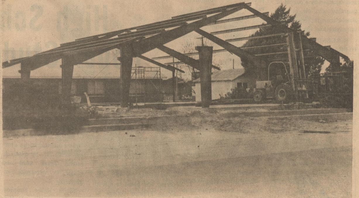
NEW CHURCH BUILDING -- Construction has begun to rebuild the First United Methodist Church in Matador. The new building will include a Sanctuary, Fellowship Hall and
