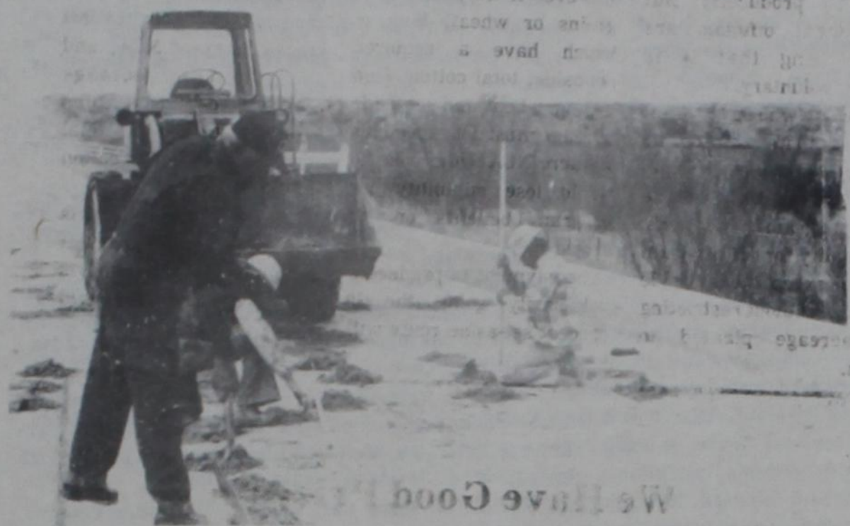
1. Demolition crew is shown above setting the charges for the blasting of the Quitaque Creek bridge.
