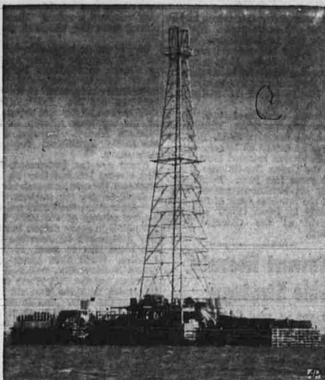
OIL WELL —Oil men from Texas and Louisiana are building this oil well on a tiny man-made island in Hillsboro Bay, seven miles from Charlottetown, capital of Prince Edward Island. The island has a surface area of 9,000 square feet.
