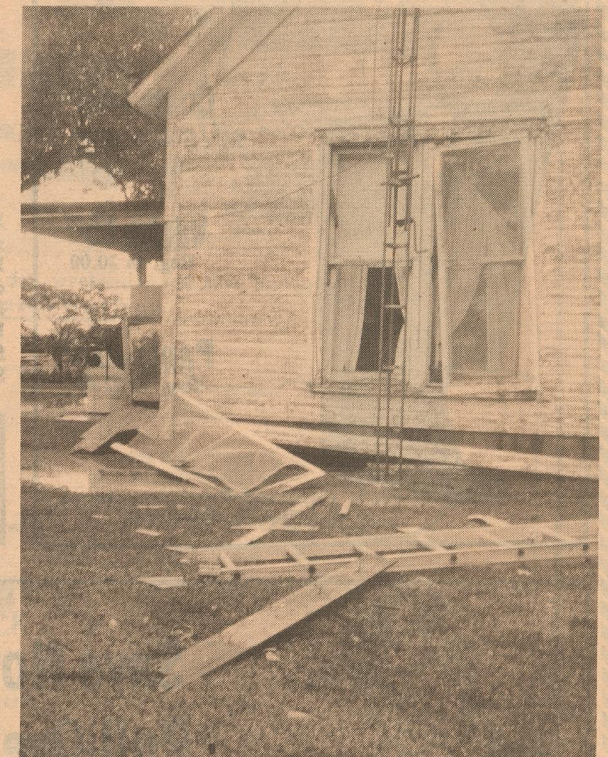
NEAR TRAGEDY - A powerful explosion ruined the inside of the Melton Brooks home, southeast of Roaring Springs, early Saturday morning, destroying furniture, dishes, carpets and even the foundation. Lightning is said to have been the probable cause, but the house did not burn because of water standing under the house left by heavy rains. Windows were blown out and the floor was buckled upward and apart in several places. The family was all in bed at the time, and no serious injuries were reported. (Photo by Gerald Garst).
