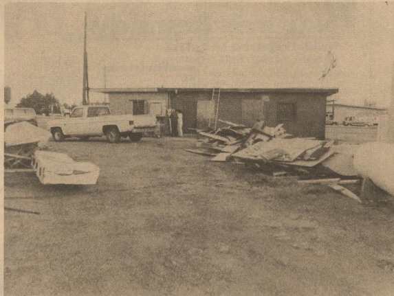
The back of Billie Dean's after the clean-up began, notice sign damaged on right corner of building. Billie Dean's roof and air conditioner united were ripped off by strong winds.
