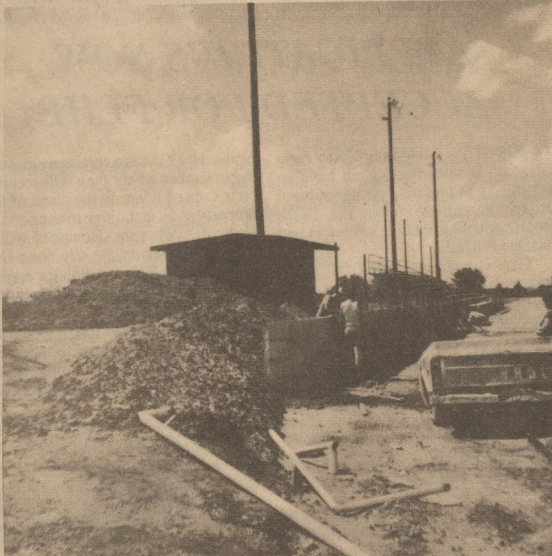
Work is being done to finish up the football/track field at the Motley County ISD Campus. Workers are building a two level retainer wall for the concession stand, foreground and pepsquad stands for the south end of the spectators stands.
