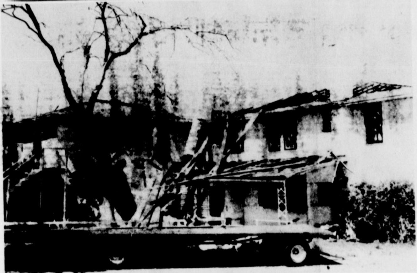
SOON TO GO -- The former Motley Hotel owned for many years by Mrs. Margaret Newman, now residing in Hamilton, and her son, the late Tom Newman, is soon to be razed. The work of removing the building is now in progress. Located at the corner of Bailey (US Highway 70) and Bundy Streets, it was built about 1919-1920 by the late Judge W. R. Cammack, and was operated by him and his wife as the Cammack Inn, until Mrs. Newman purchased it in March, 1934. Formerly, it had been a residence owned by the late Mr. and Mrs. W. W. (Billy) Moore. More recently the property was owned by Wilson Cook, who sold it to Mrs. May B. Simpson. Mrs. Simpson has sold the hotel building to Bobby Jameson, who purchased the structure and all its contents. He is to clear the lots with the exception of the small residence at the south, where Mrs. Simpson lives with her son, Fred G. Simpson. Jameson is reported to be planning to use the material for some new construction near Jameson Lake, east of town.
