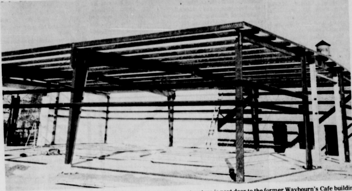
NEW BUILDING -- This picture was made last week of the Matador Motor & Implement Company's new building on Bailey Street (US Highway 70). The frame was put up one day and the building was up the next (walls and roof). The new
