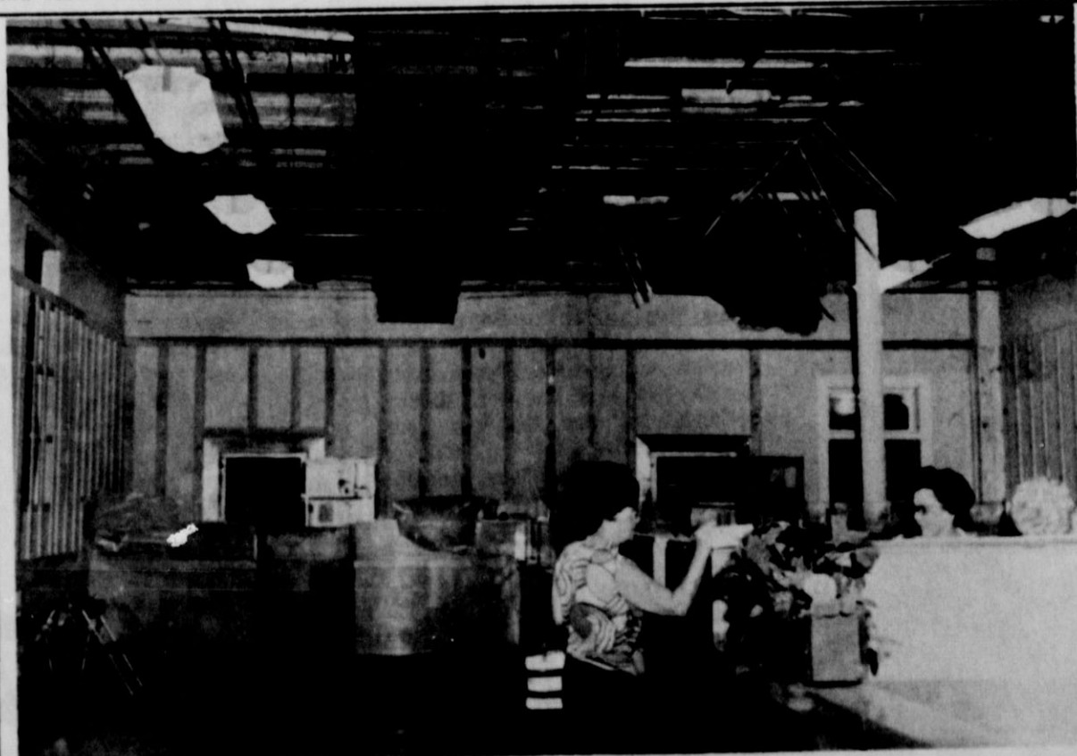
IT LOOKS DIFFERENT NOW — The First State Bank looked like this until last week end, after the extensive remodeling got under way. Since this photo was made the walls have been paneled, the ceiling lowered and new ceiling and lighting installed. The refrigerated air conditioning system has been placed in operation. The floors will be carpeted. Customer at the window is Mrs. Al Watson being served by Mrs. R. E. Campbell Jr., teller.
