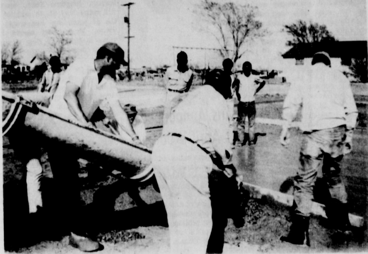
LIONS WORKING like beavers are shown above in constructing a 40x60 foot basketball court in northeast Matador near the former colored school. At the cement chute is Lion Tail Twister Glen Brotherton. The project seemed doomed to damage late Saturday when a rainstorm passed over this area and left .32-inch moisture (and some hail) on the freshly poured cement. A group of Lions went back to the project early Sunday and worked cement into the surface of the court. —Tribune photo
