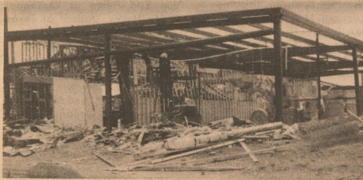
SCHOOL COMES DOWN- Through the ruins on a nearby house (top) the work crews can be seen taking down what is left of the Motley County School. The school was destroyed by a tornado on May 1, 1984. Piece by piece the workers take off twisted debris until only a frame (bottom) on the northeast corner stands above the ground. (Photo by Leon Watson)
