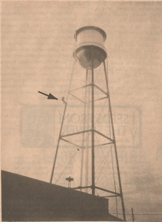
SILVER FACELIFT- After giving the inside of the Matador water tower a bath, workers last week painted the tower a shiny silver. After weeks of work the tower is ready to last years more, "we hope" before the city has to give it another facelift. This photo shows one of the workers halfway up the tower using a spray paint gun. (Tribune photo)
