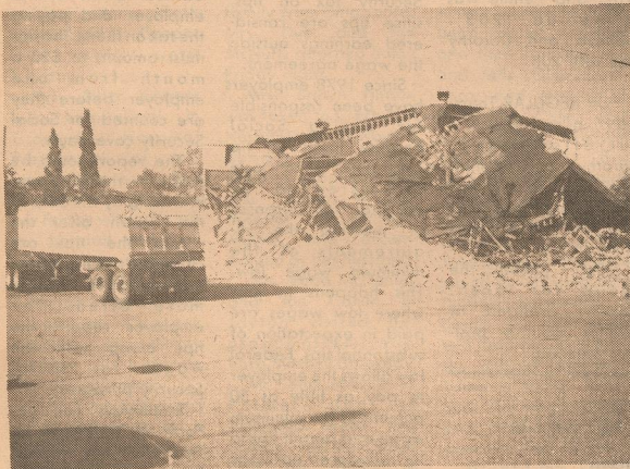
LANDMARK DEMOLISHED -- Work began late Saturday evening on the demolition of the old Matador High School building. Ray Champeau of Amarillo was contracted to tear down and remove the structure. The building had been vacant since 1974 and was considered hazardous to anyone entering it. The school building was constructed in 1925.
