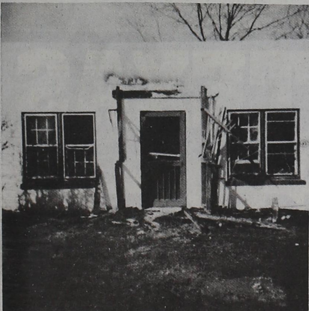
GUTTED BY FIRE — The old Boy Scout hut in Roaring Springs was gutted by fire last Wednesday afternoon, when burning trash from a neighboring building got away. The Boy Scout hut was built in the late 1940's. It has been used in recent years for ceramics work by Mrs. Georgia Witcher of Roaring Springs.
