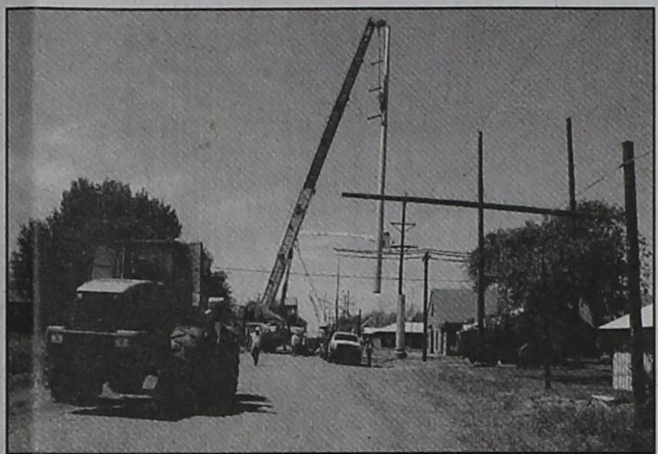
The ETT transmission line crew uses heavy equipment to place a large tower, directly south of Matador Clinic on Main and Lariat Streets. photo Carol Campbell
