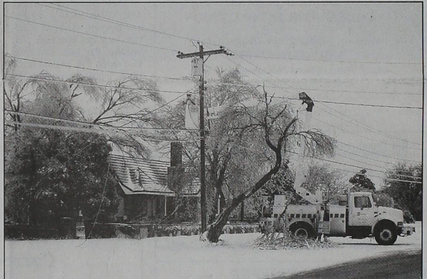
Local electrical crews worked hard on Friday to repair a downed power line due to a large tree branch that fell. AEP reported minimal power outages in Matador. (Photo by Charli Bigham).
