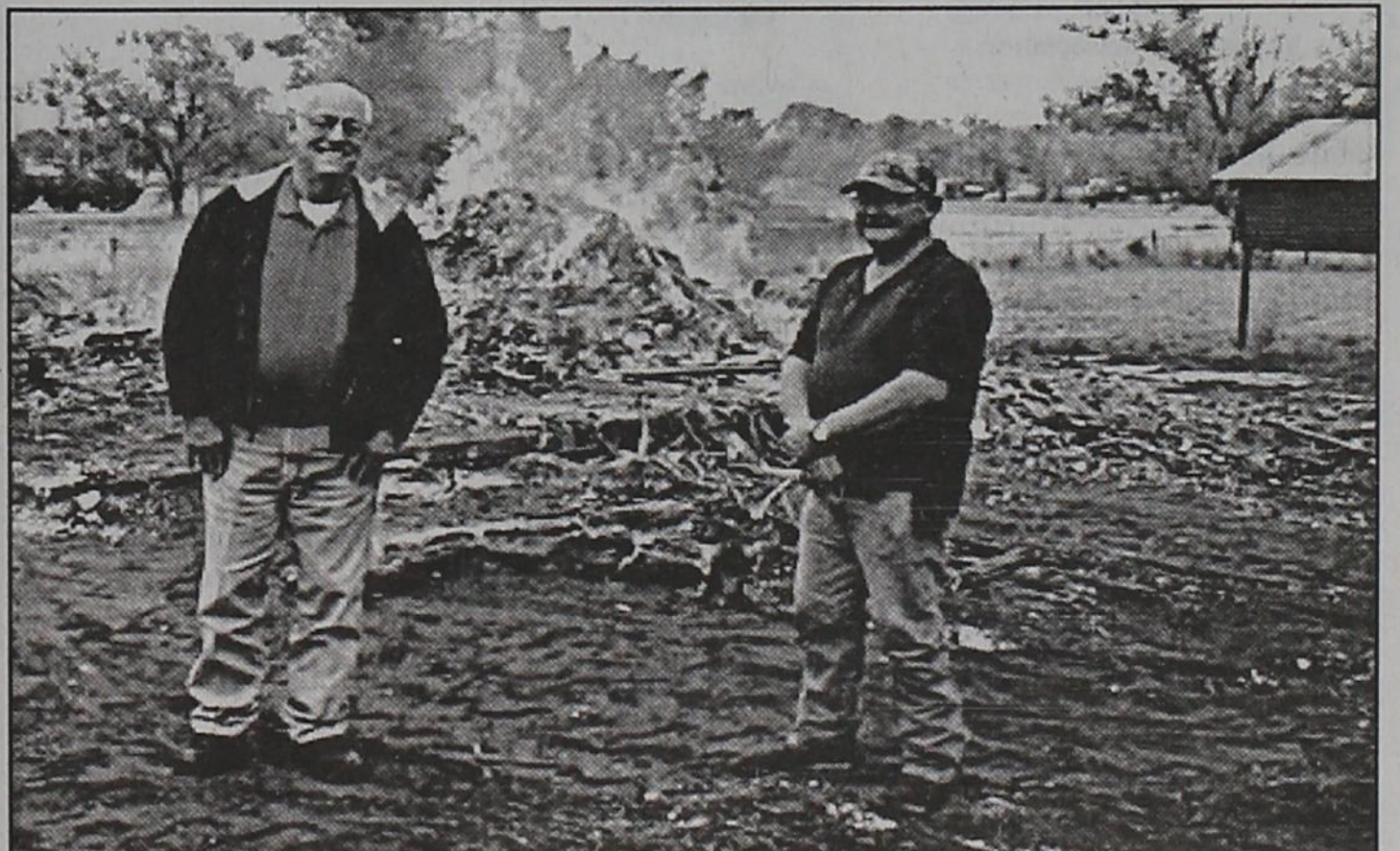
Matador City Superintendent Steve Barton oversees another old vacant house being demolished and burned. Also pictured is Ron Bailey, owner. The City of Matador is making every effort to encourage all owners of such properties to allow the city employees to get rid of them at no expense to the property owners. This is being done to make our city as clean and attractive as possible.
