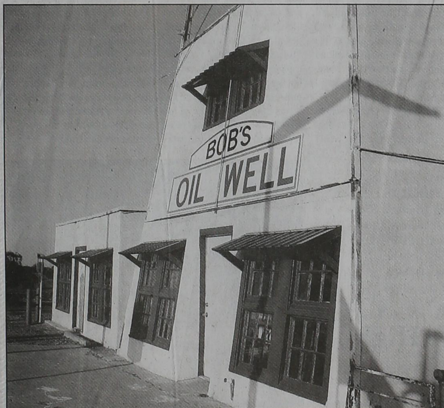
Bob's Oil Well has a face-lift just in time for Matador's Centennial. Billy Green Construction and his talented crew rebuilt window frames, painted and custom-made awnings for the windows. They had a picture to study of Bob's in the 1940s, and built window covers to resemble the early days.
