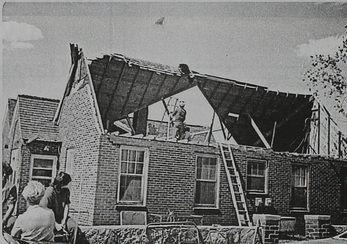
Surveying the damage, the roof covering the bedrooms in the south part of the house was lifted to oblivion, along with the brick. This 3-gabled house was pelted with golfball-sized hail tearing giant holes in the roof, and shattering all the glass. (Note the cat on the roof, taking a look into the house from a vantage point that only a cat could muster). (Photo courtesy of Bundy Hal and Dixie Campbell).
