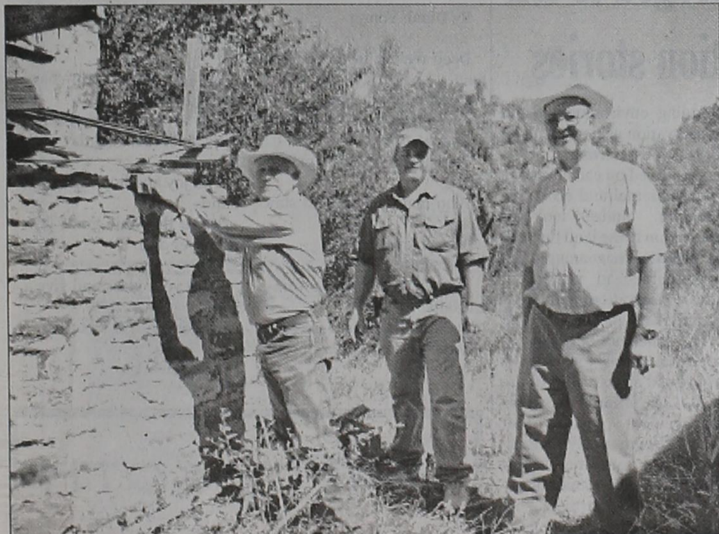
BOB KILMER, Bobby White, and Judge Ed D. Smith remove stone from the old Scotsman Dive that the Matador Ranch is in the process of dismantling. Part of the stone will be hauled to the jail location to be used as replacement stones on the roof parapet.
