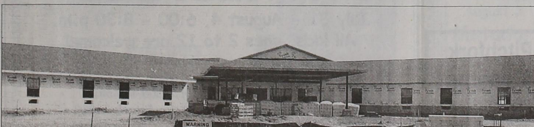
CONSTRUCTION PROGRESSING — As seen in this photo construction progress is being made everyday on the Hackberry Creek Care Center in Matador. Workers are now busy with inside work. Completion is expected by early Fall.
