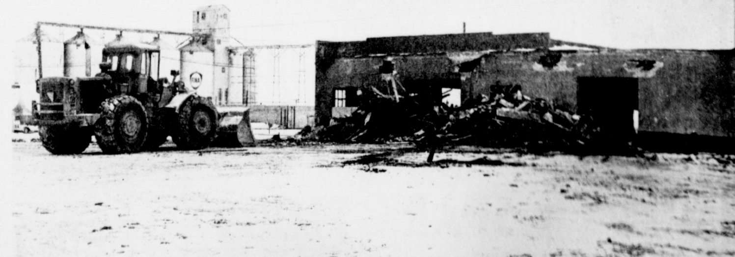
LANDMARK COMES DOWN . . . The crossroads of Muleshoe will never look the same again as a landmark was torn down this week to make room for Muleshoe's growth. The old Muleshoe Motor Company building that had stood on this particular corner for many, many years was torn down this weekend to make room for the new Muleshoe State Bank building. Construction on the new building should get underway in the next few weeks. A crowd from Jake Diel Dirt and Paving demolished the old building in just a matter of days.
