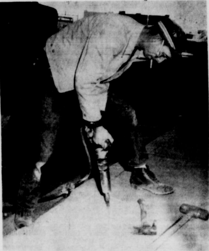
FOR FLAG POLES—Contactor Kirby Campbell is drilling a hole in the concrete in front of City Bakery. It is a part of a new plan by the Matador Lions Club to place a flag in front of every place of business on special days (First will be Lincoln's Birthday, Feb. 12). A special Lions committee will place a new flag in each iron pipe holder sunk in the concrete.
