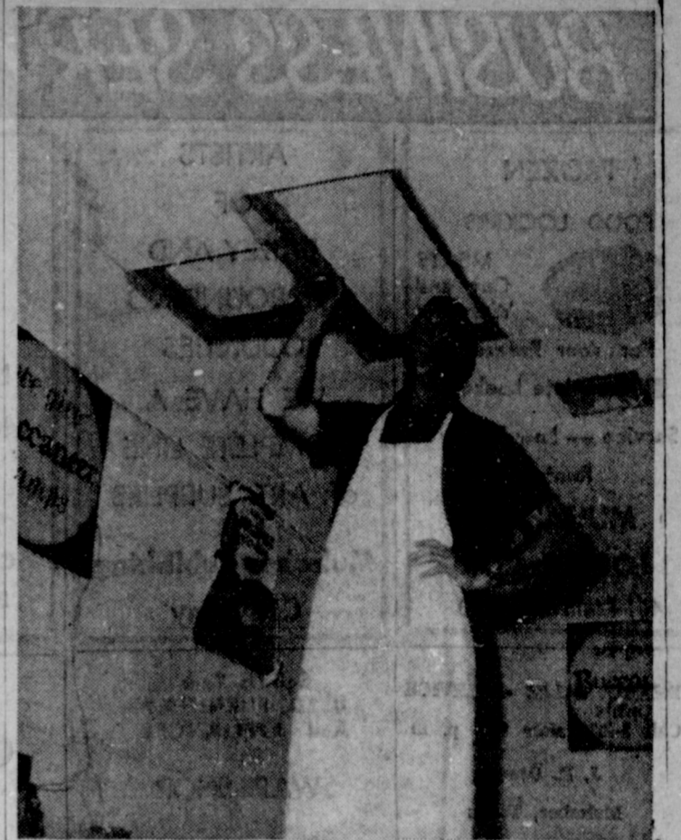
BILL MORRISON SURVEYS the damage done to the ceiling at his store when burglars entered his store some time Tuesday night. Total loss was reported to be around $100 by Morrison.
