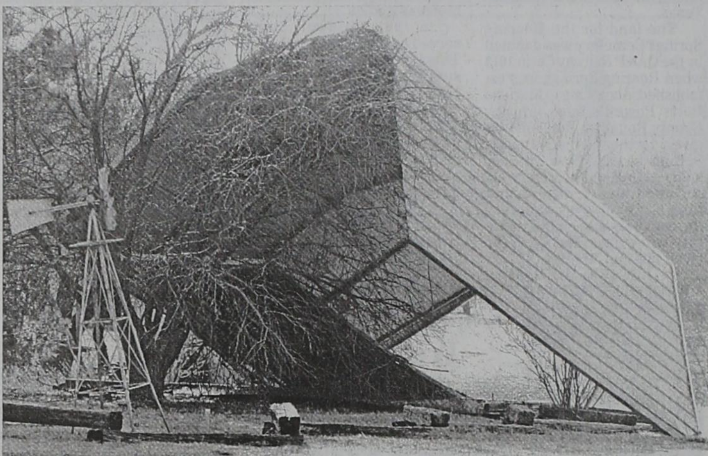
WIND DAMAGE — This carport at the home of Sammie Phillips in Matador was overturned and damaged by the high winds in Motley County last Saturday, February 24.
