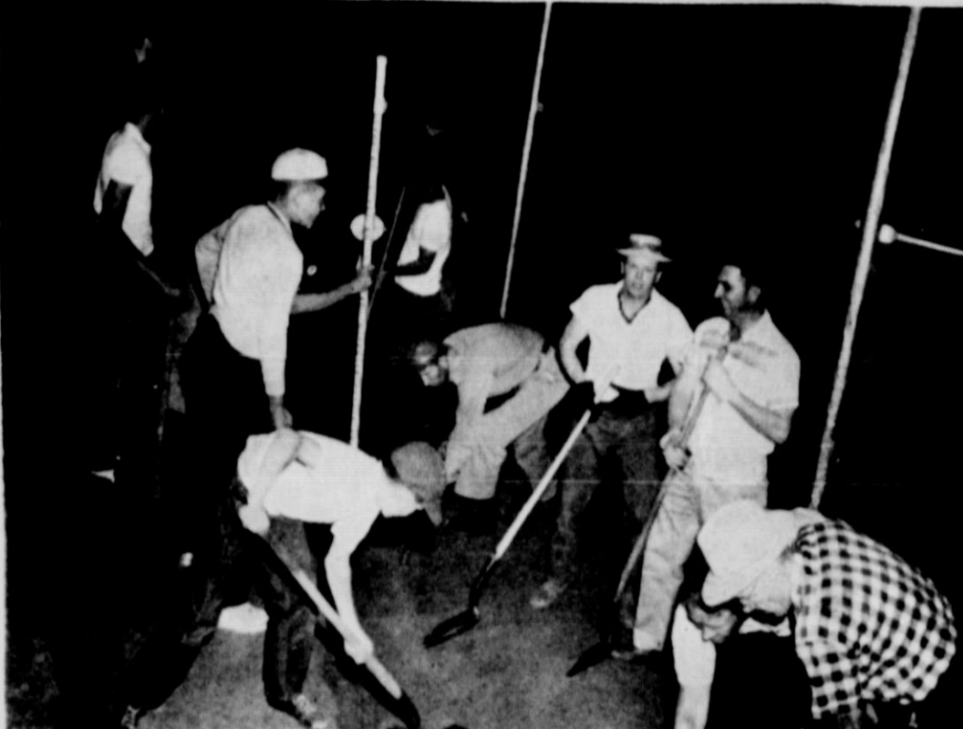
WILLING VOLUNTEERS — More than 20 men and boys reported for work at the Matador Baseball Park Friday evening as construction of the concrete bleachers was started. In addition to the volunteer labor, several power machines were brought into use, including the City of Matador's new back hoe and loading machine, operated by City Water Superintendent Sonny Jackson. In above photo VFW Commander Richard Turner (wearing hat) and Billy Wason rest their shovels a moment. At extreme right is R. E. (Pappy) Campbell, who is an avid baseball fan. Immediately back of him is L. M. Cox.
