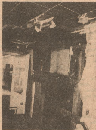
These charred walls and ceiling tell the story.
