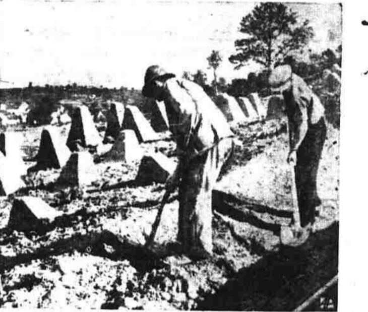
THEY SHALL NOT PASS , decided Germany, thinking of enemy tanks, and so teeth-like concrete blocks designed to rip off tanks' caterpillar treads supplement the Limes steel and stone defenses. The fortifications, built to match France's Maginot line, is to be finished this winter.
