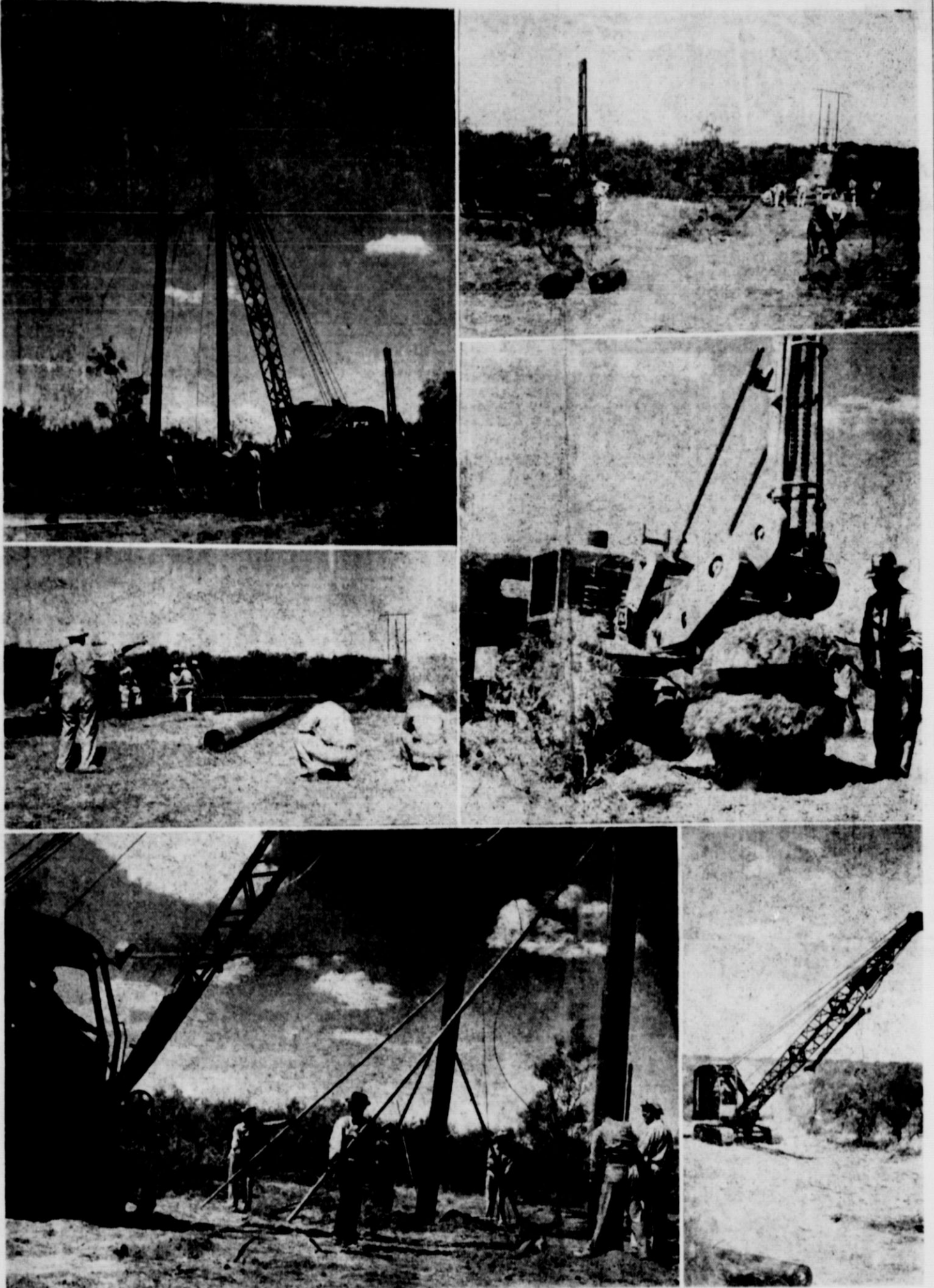
END OF A RUGGED TRAIL is shown above as the West Texas Utilities Company's new 66,000 volt power line "loop" nears completion, west of the Matador townsite at U. S. Highway 70. Upper left picture shows the last "H" frame on the 28-mile line from Turkey being set into position with the setting crew holding the 50 to 65 ft. poles for exact positioning. The poles are placed from 7 to 8 feet in the earth. The "H" frame is held in position by the drag line. Wires dangling from pole are not power lines but guy wires which will be secured to "dead men" and hold the "H" frame against heavy stress of lines. Second picture, top right, was made before the frame was raised and shows framing crew at work. Note bladed trail across mesquites and "H" frame being raised in the distance. Two short creosote poles in foreground are "dead men" to be buried to anchor "H" frame which is still on the ground. Center left picture shows D. L. Moreland, digging machine operator for Allhands & Bailey of Dallas, contractors for the line erection, signalling the drag line operator, in straightening the "H" frame in the distance. Right center picture shows operator Moreland digging holes for the "dead men". The machine digs a 20-inch hole 7.8 feet deep in one minute and 45 seconds. Bottom left shows Odie Qualis holding the frame in exact position. Lower right picture shows the heavy frame a fraction of an inch. Setting crew is holding the frame in position until they have been dragging the line moving up to set the last frame. Note dangling "spreader" which holds the poles in position until they have been anchored. Pictures were made on D. L. W. Birnie land west of town. The digging machine did not bring up any moisture when anchored. Pictures were dug. R. N. Jackson, superintendent for Allhands & Bailey, whose contracts frequently include the construction of railroads and highways, said that in his 25 years experience, the terrain between Turkey and Matador was the roughest he had ever encountered. In places the work required two drag lines and two "cat" tractors. The new line when it is placed in operation, will give Matador electric current that might be used to serve a city the size of Abilene. Cost of the line is estimated at $145,000, bringing "loop" service to Matador, Turkey, Paducah, Estelline, Caray, Childress, Goodlet, Quanah, Crowell. "Loop" service means that in event of interruption of service from one direction, current can be delivered from the opposite direction in a few moments.—Photos by Douglas Meador.
