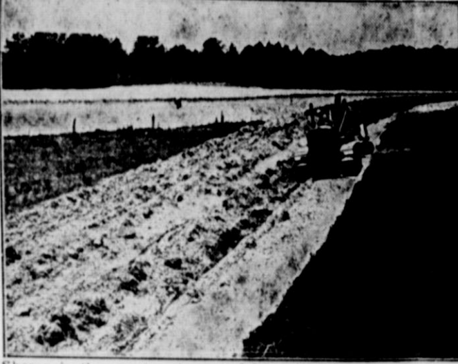
Shown is the construction of field terraces, similar to the 125 miles of standard large ridge type terracing completed in Motley County. Time for winter terracing has arrived, according to
