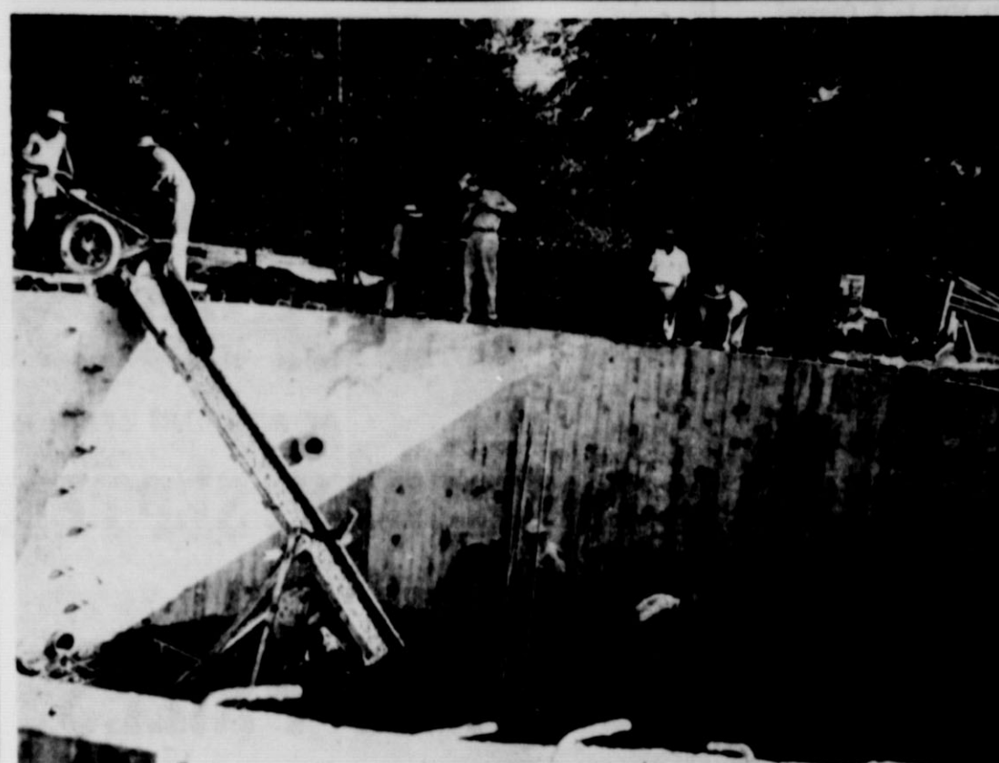
POURING FLOOR to city of Matador's new 100,000-gallon water storage tank. Left to right two unidentified Negro workmen, City water superintendent Herman Stanfield, Councilman Joe Campbell (standing on rim of tank), engineer Cecil M. Hawk of Lubbock and E. K. Hester (looking down at other workmen smoothing floor). Contract for the big steel reinforced concrete reservoir is being completed by the Hester Construction Company of Lubbock. The roof has now been completed and connections made. Last night the tie-in was made between the new reservoir and the old one of the same capacity. Curing process of concrete will require about two weeks, when tests will be made and final use in the city water system effected. When the tank is placed in use the municipal water system will have 250,000 gallons reserve, in addition to storage in mains. (Photo by Douglas Meador).
