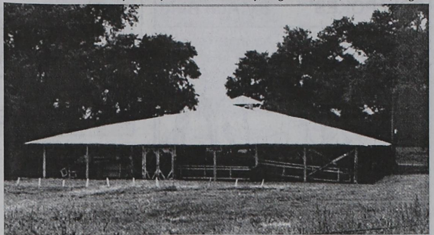
The historic Old Settlers Tabernacle is in dire need of major repairs.
