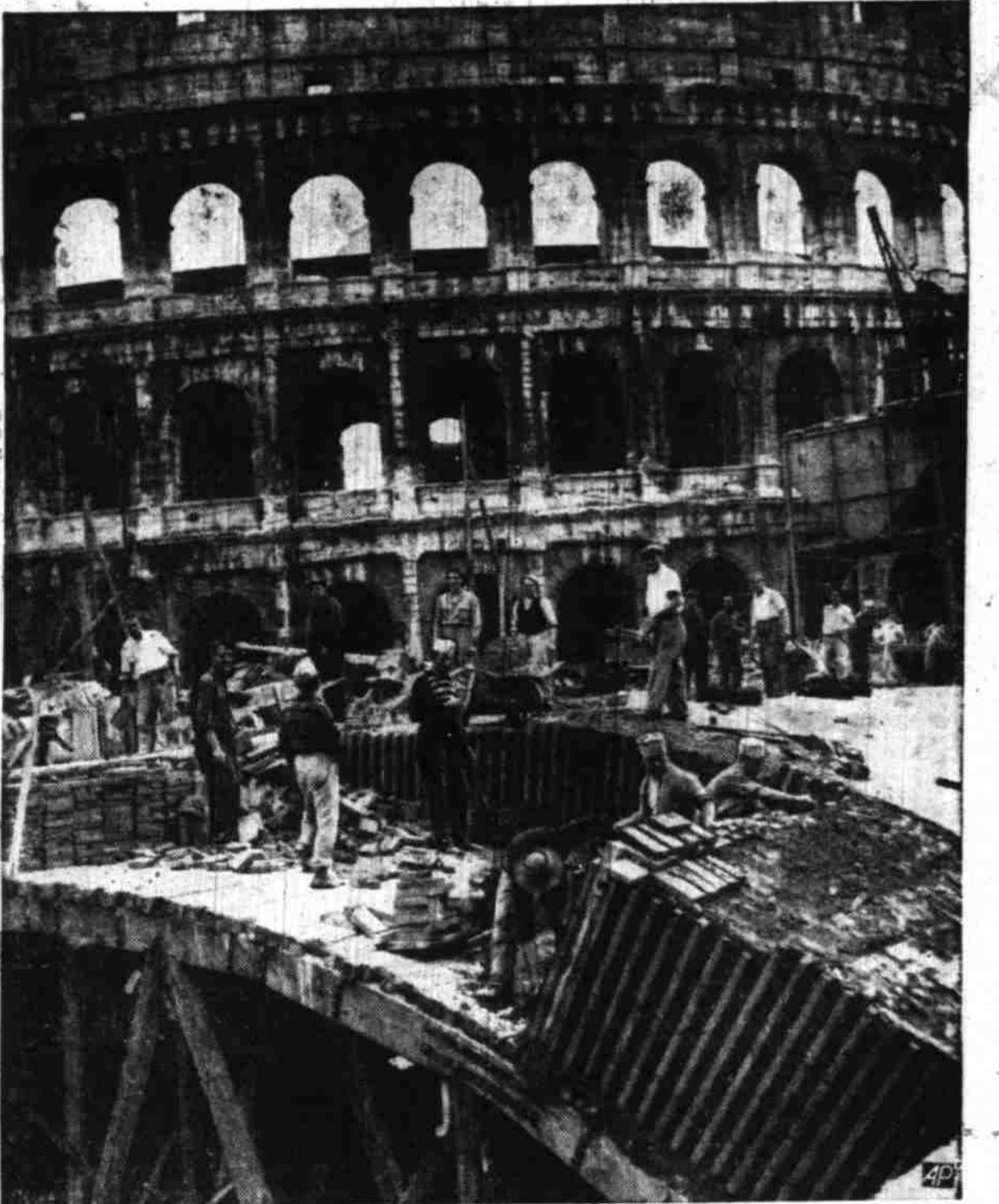
SUBWAY BY COLOSSEUM —Close by the historic Colosseum, Rome workmen are constructing a subway which will extend from the central railway terminal to St. Paul's gate.
