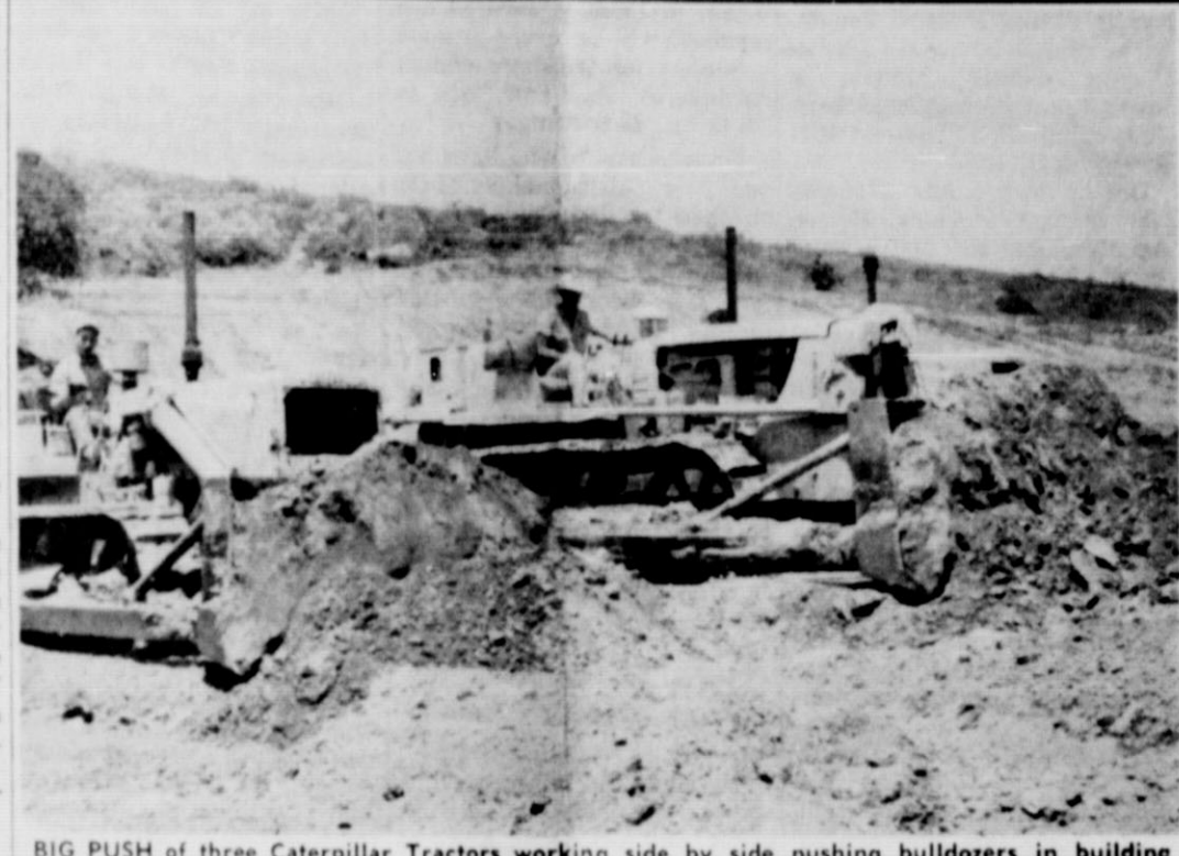
BIG PUSH of three Caterpillar Tractors working side by side pushing bulldozers in building a dam on the Robert Reynolds farm in Dickens County. The dam in the above photo contains about 6,000 cubic yards of dirt, and was built where a smaller dam had formerly washed away. Two other large dams were built on Mr. Reynolds' farms in the Croton Flat area. The water conservation and flood control work was done by Price Construction Co. of Snyder.
