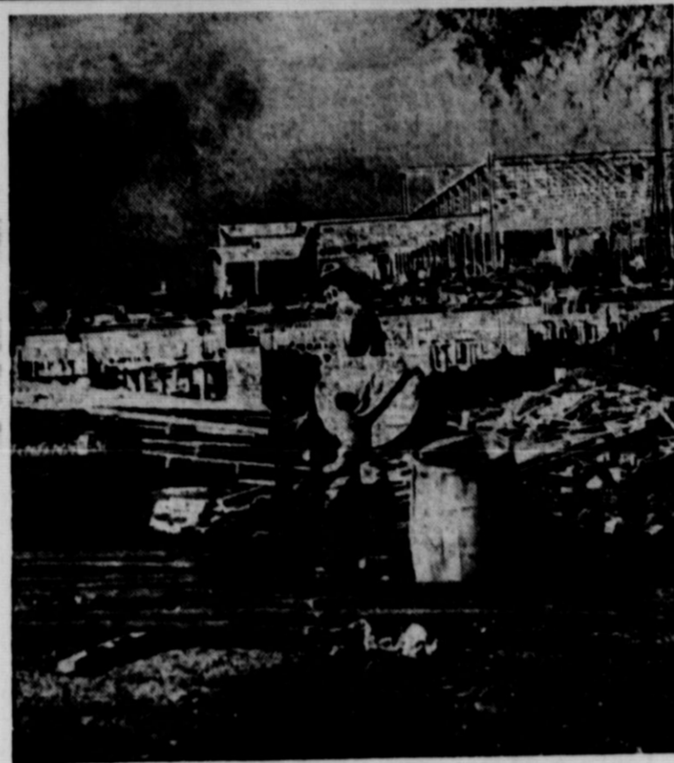
The steel frame of the $140,000 Livestock Building No. 2 for the Texas Centennial Exposition at Dallas can be seen above as it rapidly takes form. With the $260,000 Livestock Building No. 2 soon to be started, it will house the greatest exhibit of livestock in the nation's history when the Exposition opens June 6.
