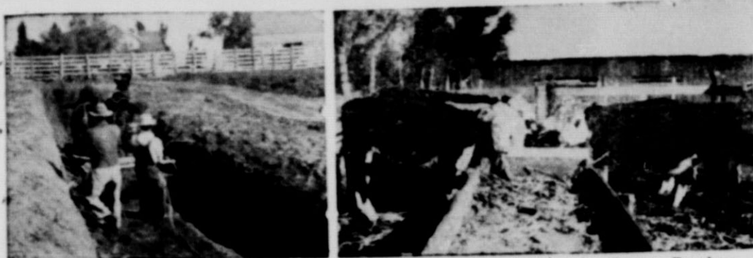
Trench silos became common in the Texas A. and M. College Extension Service District 2 as the number increased from 703 in 1936 to 1,542 in 1937. This one is being dug by U. L. Wille on his place near Matador in Motley county. Right, these 10 yearlings owned by George Branham, Jr., are part of the Hale county 4-H club boy's feeding project, which involves 200 beef calves and 500 sheep.
