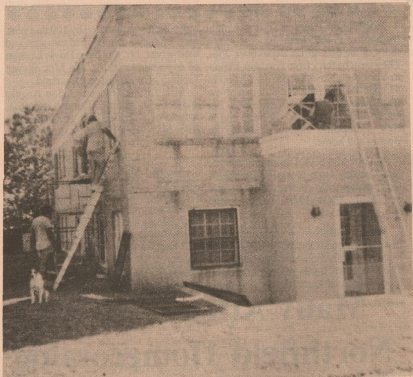
Work has begun on the restoration project of Traweek Hospital building for the Motley County Museum. Shown working is Meredith Construction crew.
