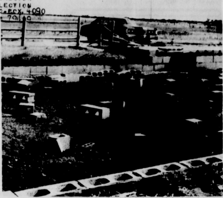
FOUNDATION LEFT - Once the foundation for the home of Leland Wood, bricks were scattered after the twister lifted the house from its foundation and ripped it apart. Leland Wood car is in background. -Photo by Mary Woosley
