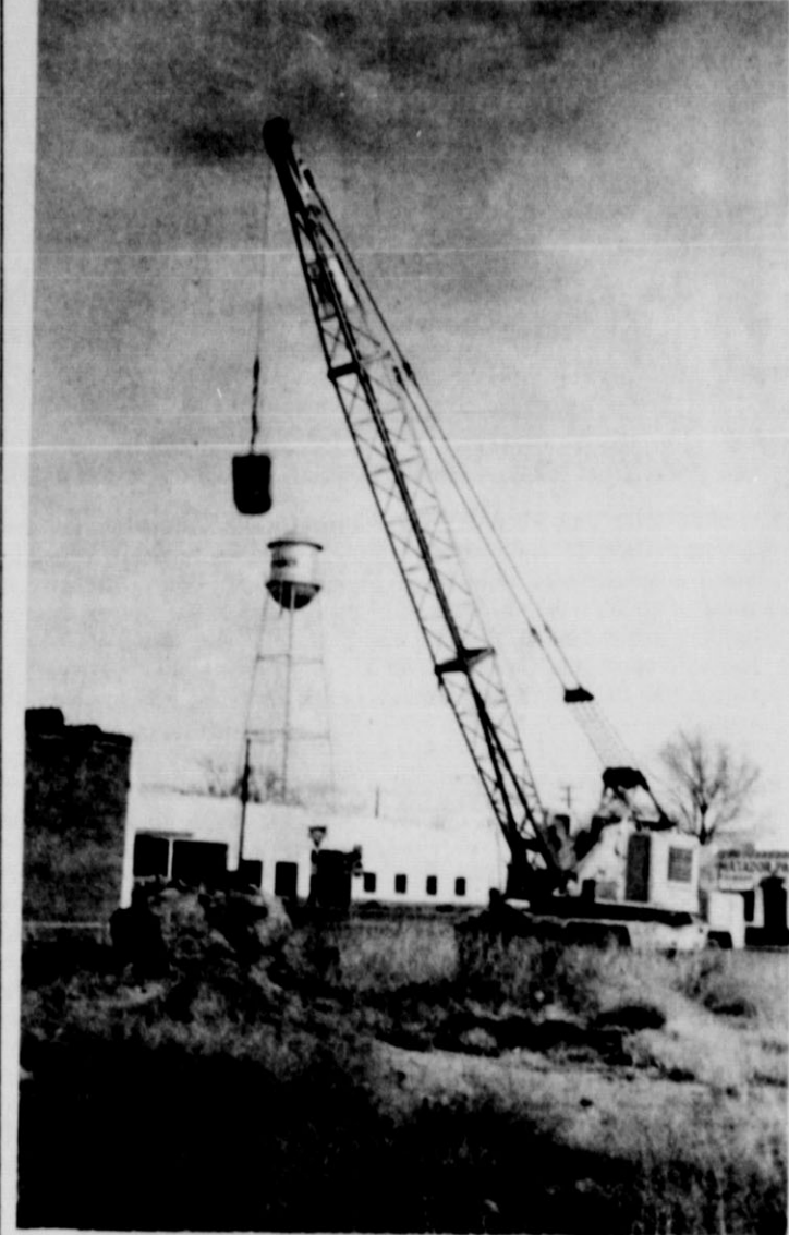
BIG HAMMER BEATS a big man-made rock on the Matador Auto Company property south of the agency. The 3000-pound weight was dropped on the steel-reinforced object until it was reduced to particles small enough to be moved with conventional equipment. This area will be leveled and used as an automobile store lot. Originally the piece of concrete had been the base for a compressor when an ice factory occupied the property. —Staff photo
