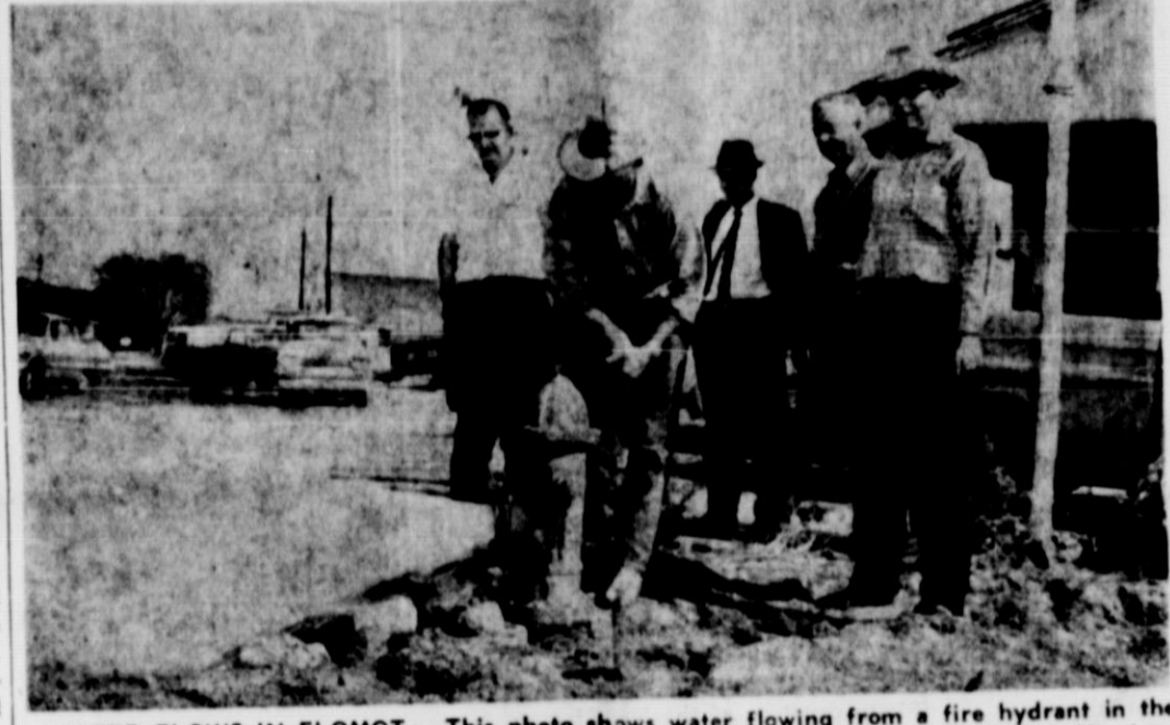
WATER FLOWS IN FLOMOT — This photo shows water flowing from a fire hydrant in the business section of Flomot Saturday morning. In the picture, from left to right are Harrison George, Wendell Morris (turning hydrant), County Judge Elbert Reeves, Sam Ross and FFA Supervisor for Floyd and Motley Counties, Alfred A. Harrison.
