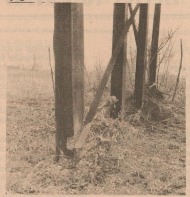
SOUTH PEASE BRIDGE: Holes rusted at base of pilings under bridge closed by state.
