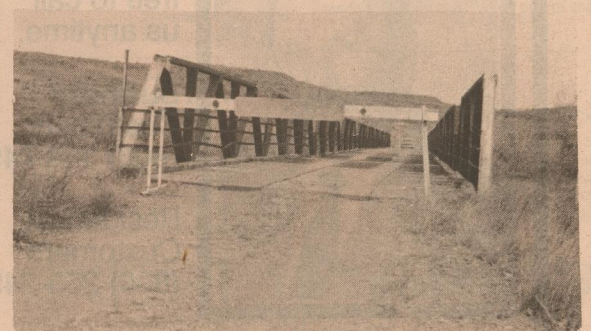
SOUTH PEASE BRIDGE approximately 200 feet across South Pease River in southeast Motley County on the county road to Dumont.
