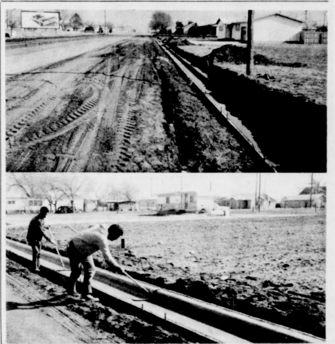
PAVING project is underway on West Lockwood. Plans call for a width plus curbing and gutter. Construction is City-State improvement project. News Photo
