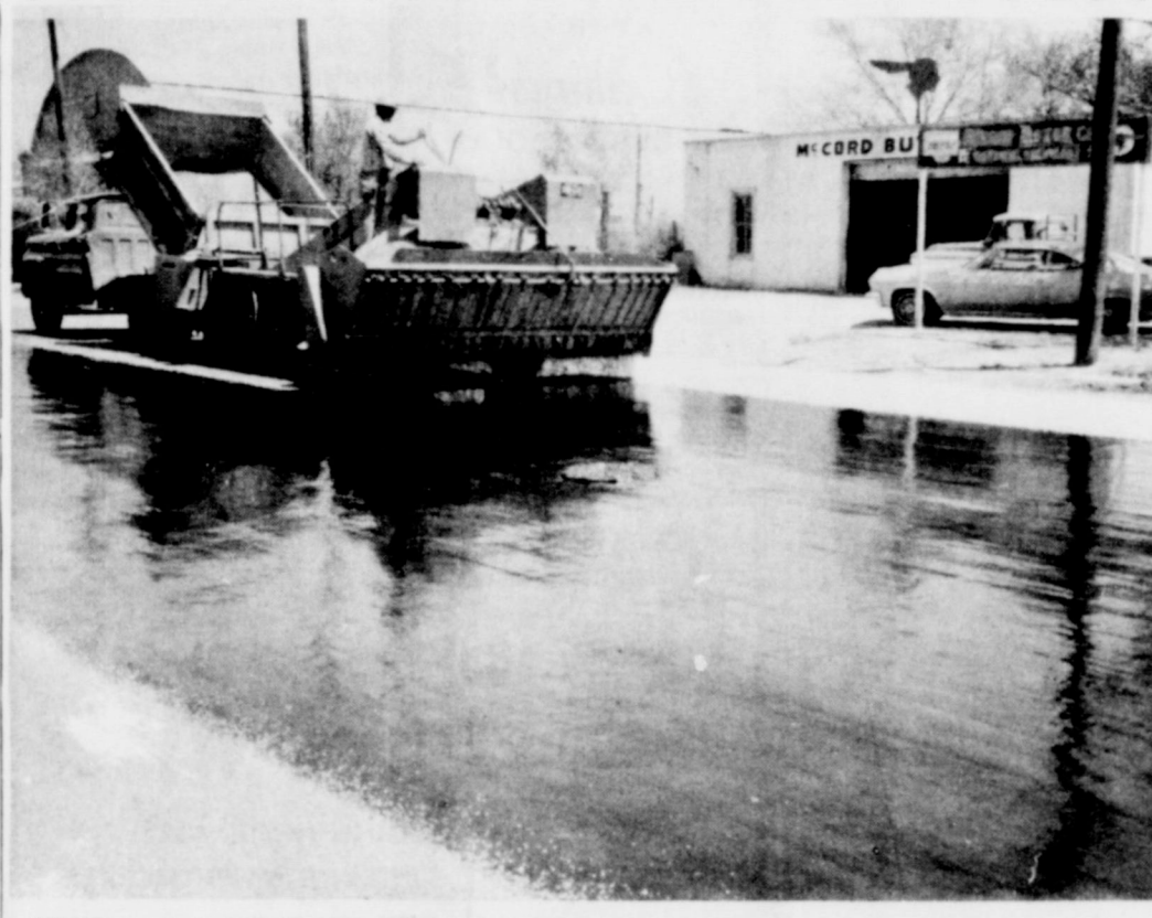
FIRST the hot stuff, then the chips. This is the makings for a new topping on Tahoka's streets. Several streets have been finished this week.
