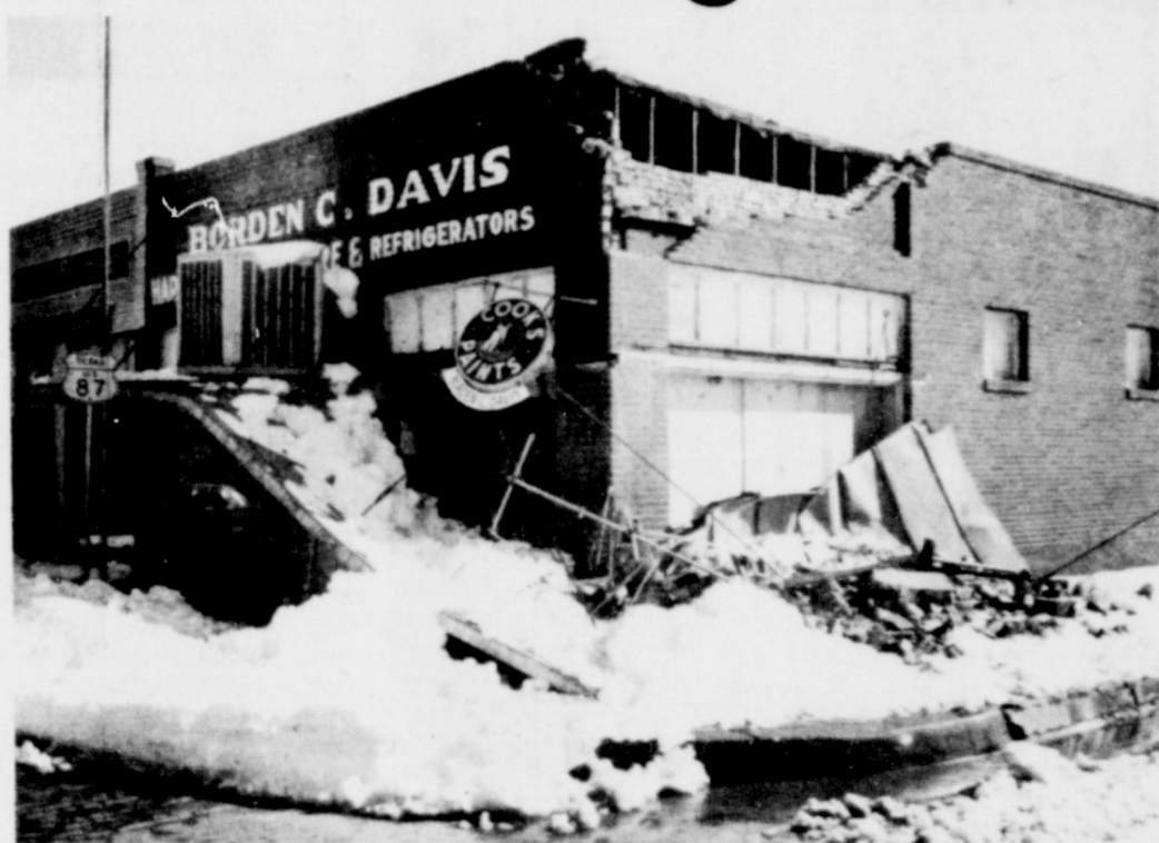
MAJOR DAMAGE resulted to the southeast front of the Borden Davis building when weight of snow piled-up caused the awning to collapse and taking a part of the brick wall with it. Only other damage reported to The News included a few leaking roofs and chug-holes in city and farm-to-market road pavement.
