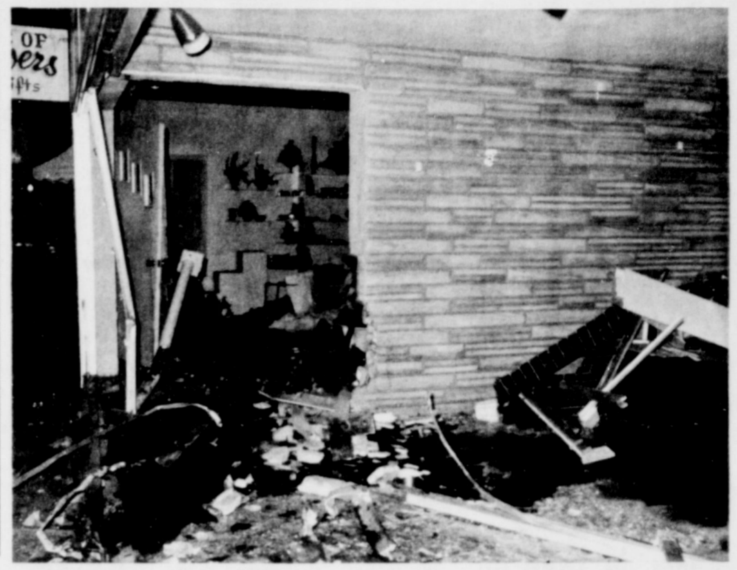
LESLIE JONES was slightly injured Tuesday night, when mechanical failure forced his 1955 Chevrolet into the front of the House of Flowers. Top photo shows extensive damage to the glass front and interior of the building. NEWS Photo
