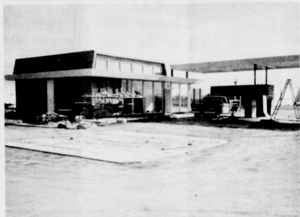
E. T. CLOE, is building this new modern Texaco station in Tahoka, at the bypass and Post Highway. Bobby Jolly will operate the station, when it opens in about three weeks.
